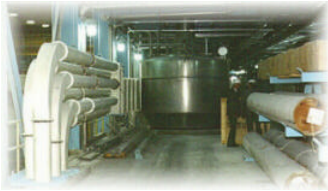
Figure6:Six Winders are Connected to this Single Bervac System
